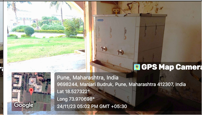
Drinking Water Cooler
